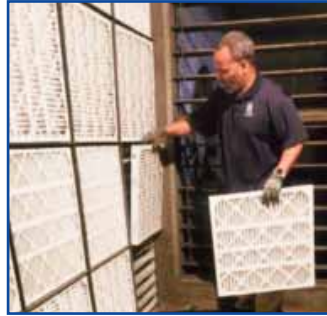
MECHANICAL SYSTEMS MAINTENANCE
