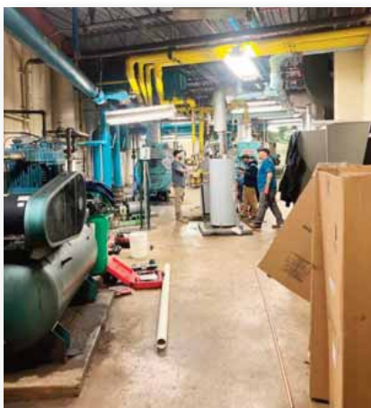
New hot water tank installed at the Ted Scott Campus.
