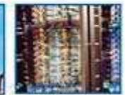
Data Center and Cybersecurity
