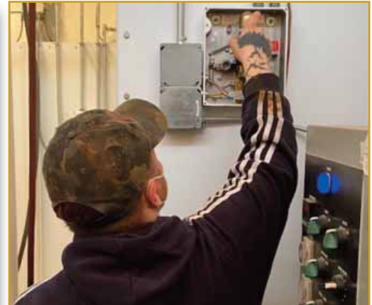
Paint booth fire suppression inspection
