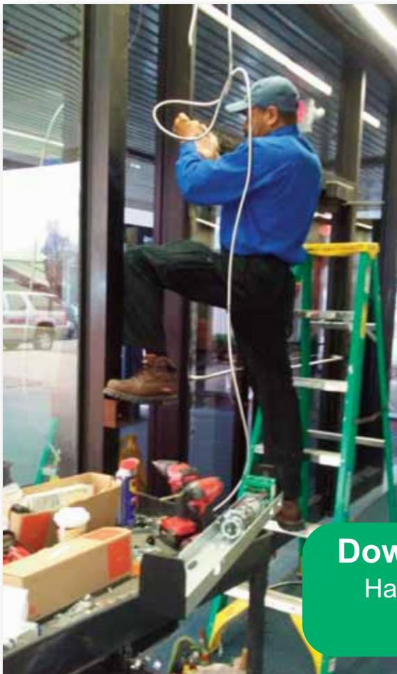
Downtown Campus and Northwest Campus Underground Lighting
