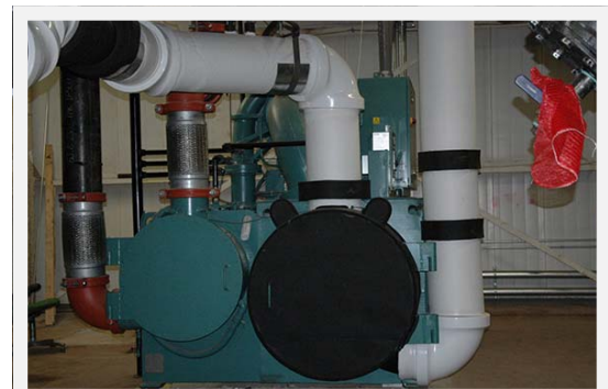
Piping into new boilers and chiller
