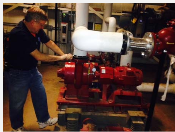
Maintenance of heating pumps
