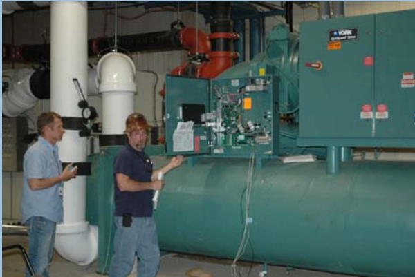
Final preparations and inspections are made for start up of new water cooled chiller at the Downriver Campus
