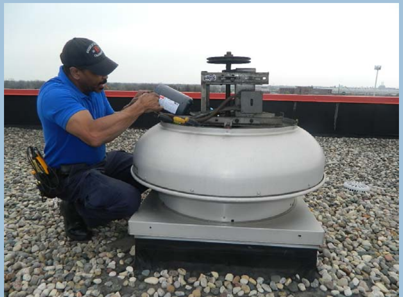
The main restroom exhaust fan motor was repaired at the Corporate College at the Eastern Campus.
